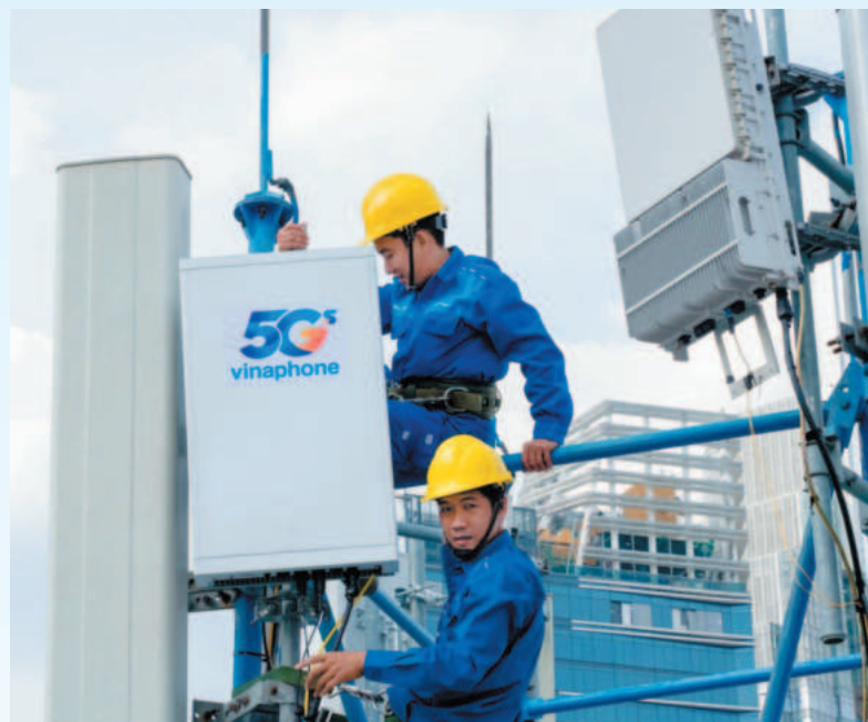
VNPT engineers are engaged in deploying operations at a 5G network station
